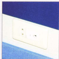
NETWORK, TELEPHONE & ELECTRIC SOCKETS
